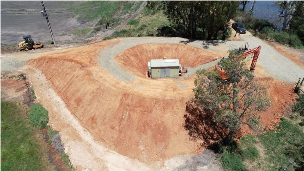
Figure 3-12 Cowirra pump station with temporary levee (preflood)
