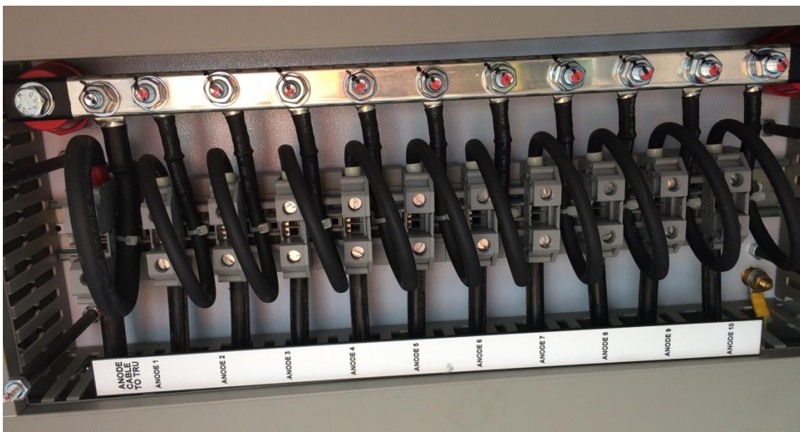
Figure 5-4: Cables within anode marshalling panel, each corresponding to a different anode.
