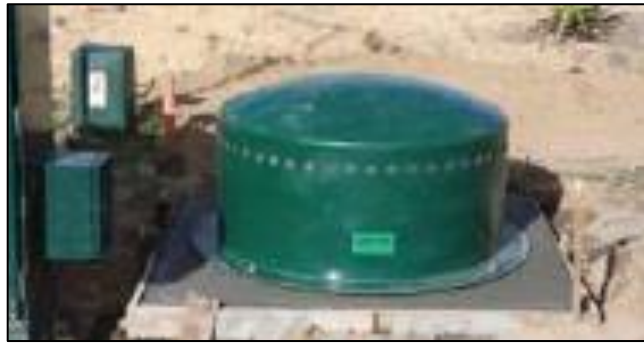
Figure 4-4 Low Pressure Carbon Filter (Green Dome)
