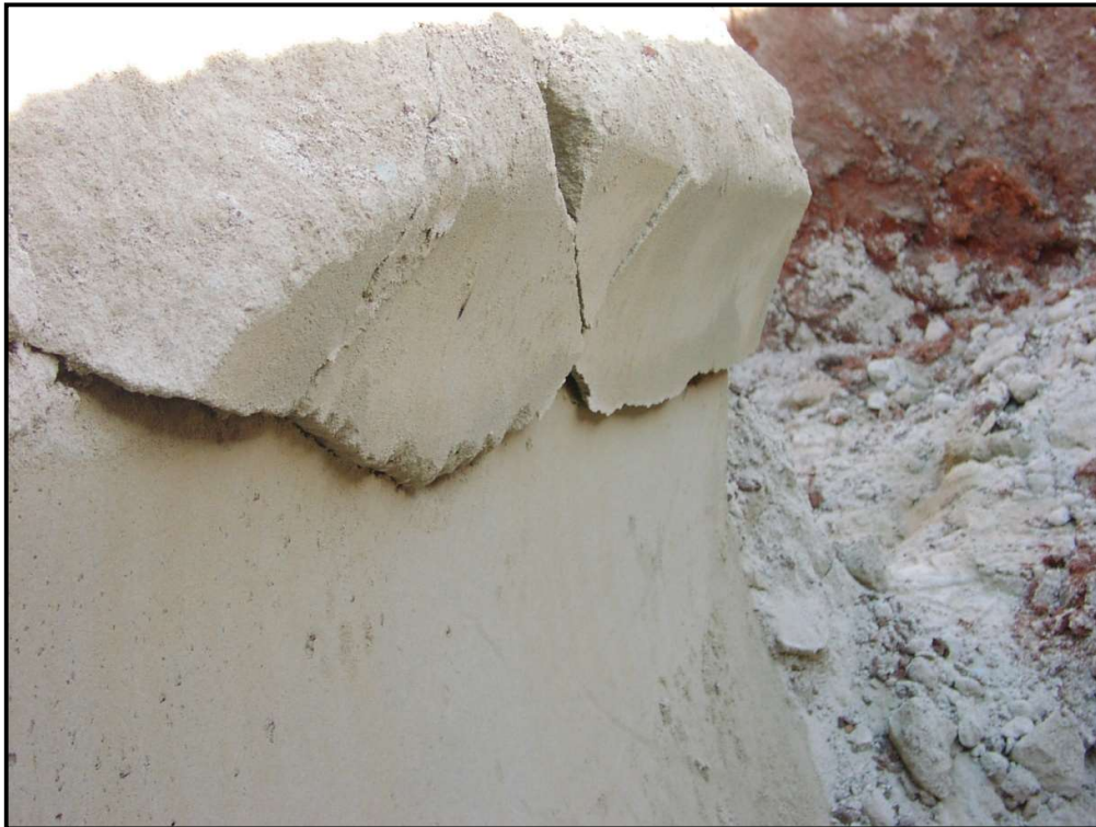
Photo 5: These lumps were above half height and broke off as the pipe was removed. A lump of the cured CLSM could be “broken with difficulty by hand” indicating a compressive strength of about 1 MPa.
