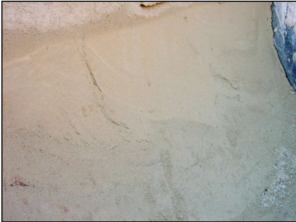
Photo 2: The left side – not vibrated. Shows “flow banding” but otherwise full contact with the pipe.
