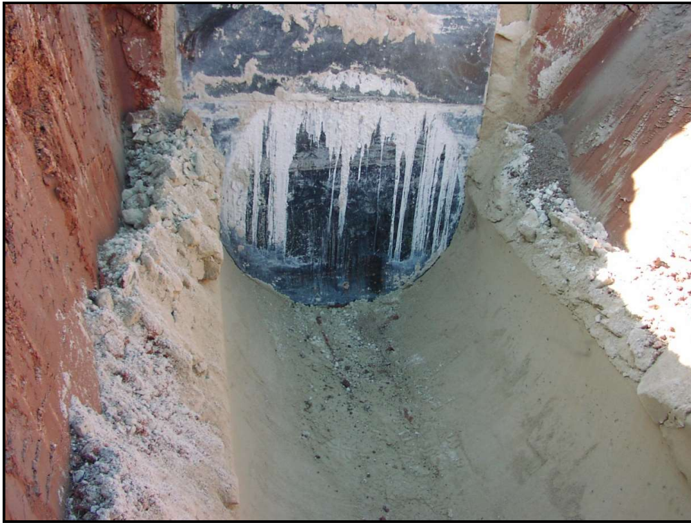
Photo 4: The CLSM made full contact with the bottom and sides of the pipe.
