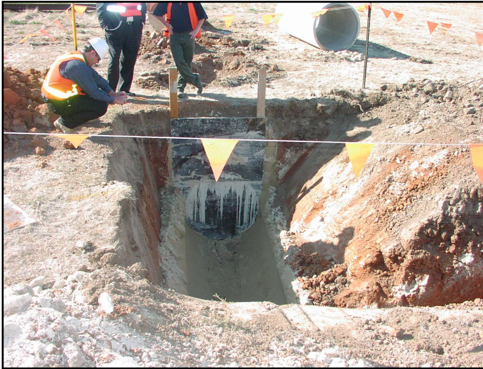
Photo 1: A concrete pipe (background) was placed in the trench and the CLSM poured to mid-height. The CLSM was vibrated on the right-hand side of the trench but not on the left. The pipe was removed when the CLSM had cured, revealing the quality of the contact.
